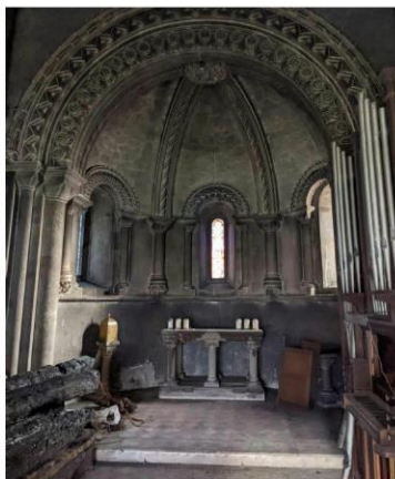
Sanctuary with Smoke Damage
